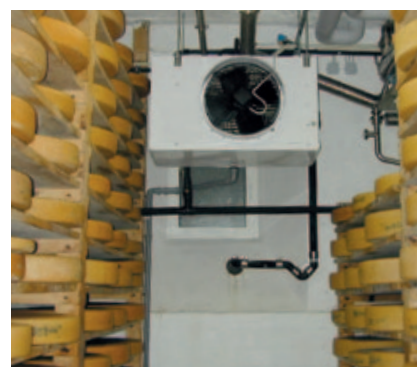
Every cheese matures at the perfect pace when the storage room is evenly cooled.
