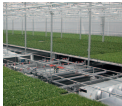
Greenhouse cooling using Alfa Laval air coolers.
