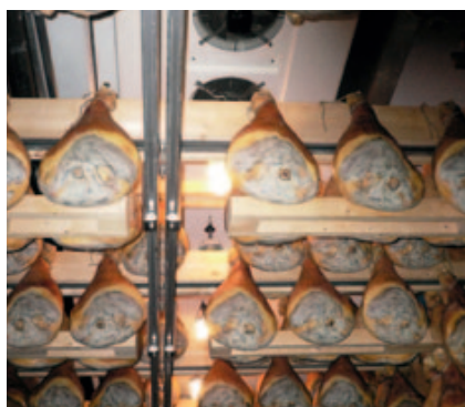
Italy's famous Parma ham is kept in perfect condition with Alfa Laval air coolers.
