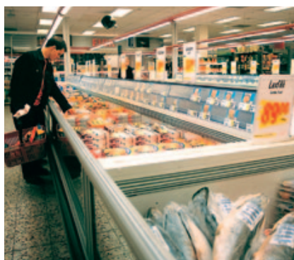
An dual-circuit cooling system keeps cold cabinets and freezer cabinets at the right temperature for each.
